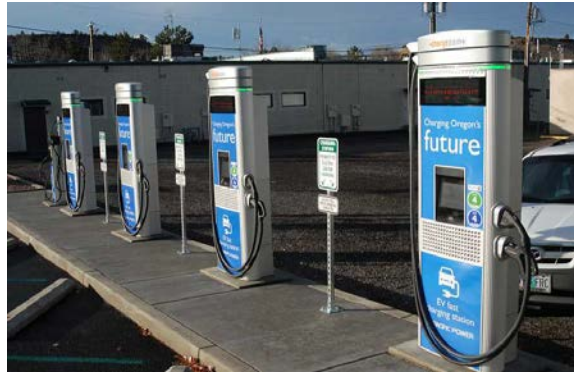
Figure 29. Pacific Power Public Charging Station (Courtesy of Madras Pioneer)
