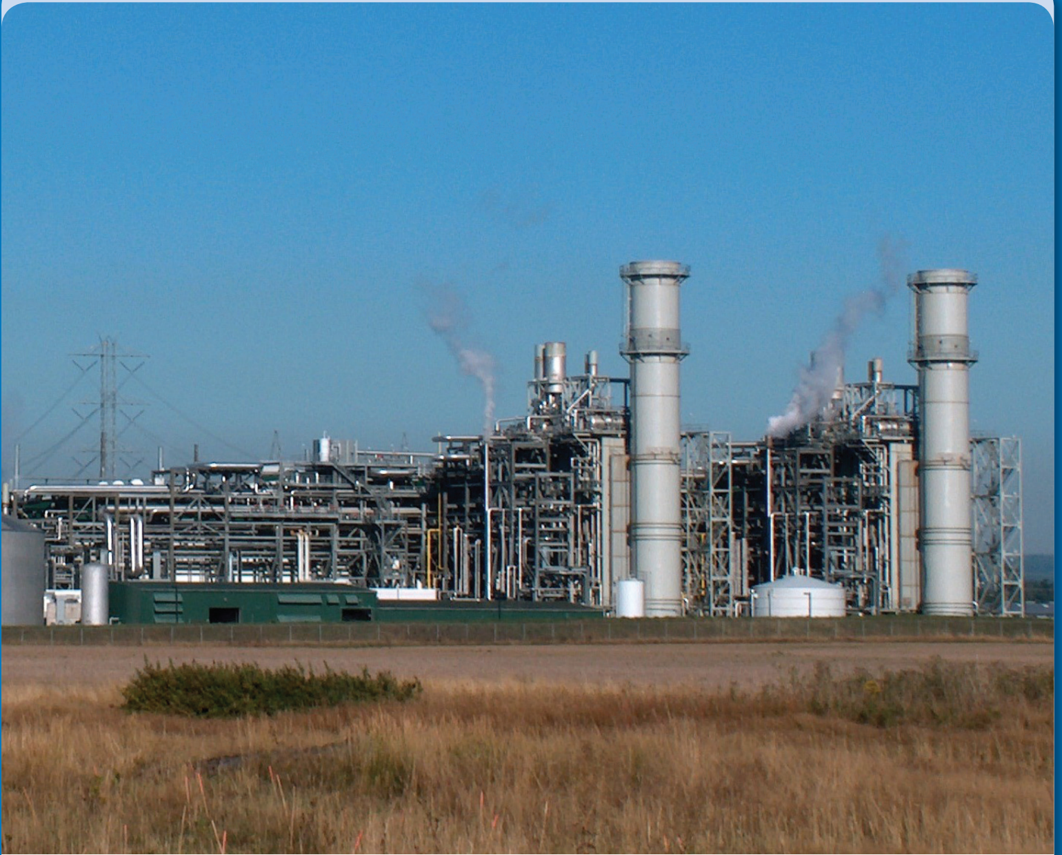
Chehalis Generation Facility
