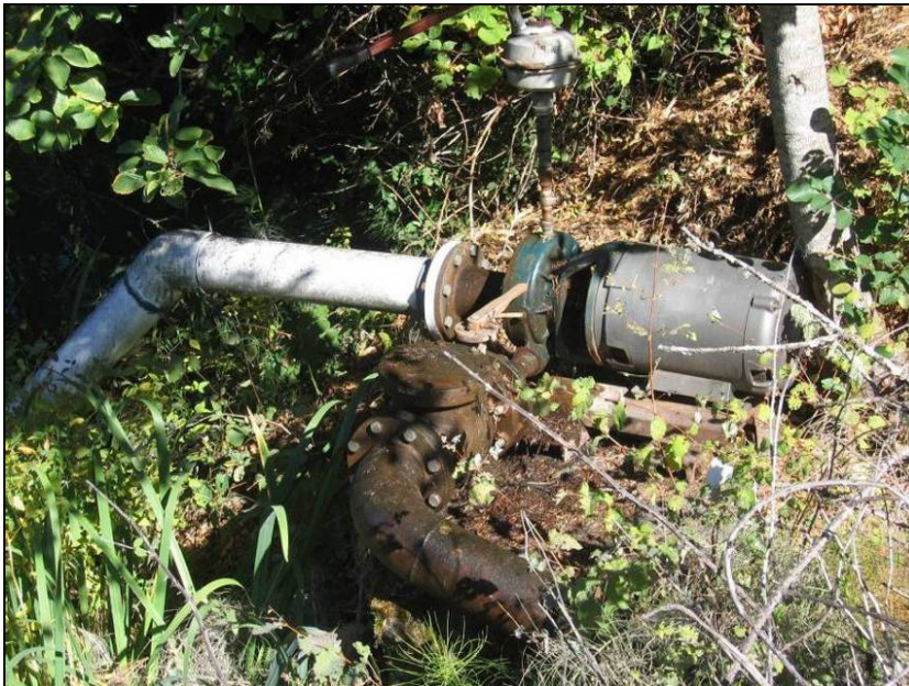
Figure 2-1 Existing Mount Adams Orchard Irrigation Pump and Motor
