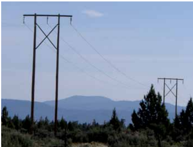
A typical wood pole 230kV structure that will be used in the new transmission line project.
