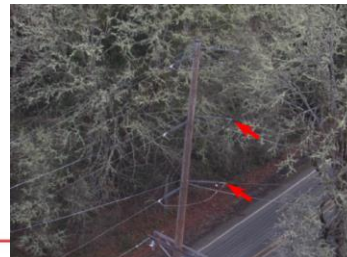
230kV Jumper Connection
