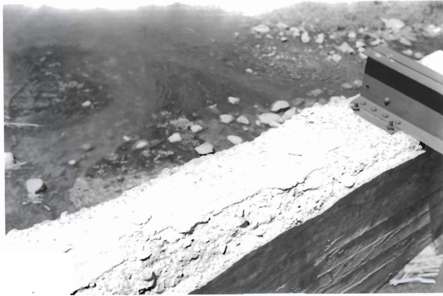
7. Showing deteriorated condition of concrete superstructure. 5-22-51
