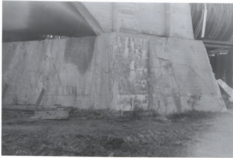
Downstream abutment right tangent. Shows spalled concrete before chipping. 8-15-52
