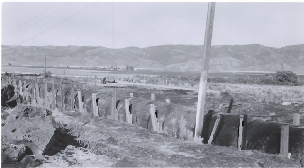
Steel section of Flowline 1 crossing over Flowline 2 after filling. With 16 to 18 ft. static head steel rounded up, releasing pressure against side braces, and allowing them to tip over. Top tension rod prevented loosened sets from falling completely away from pipe. 7-27-48
