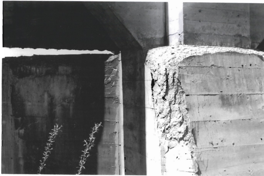
4. Showing deteriorated condition of concrete superstructure. 5-22-51
