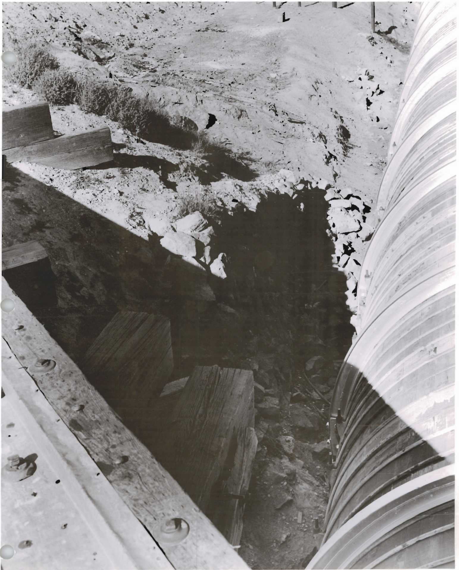
U.P.R.R. CO. Bridge over Grace Flowline, showing dry masonry No. side and pipe looking upstream
