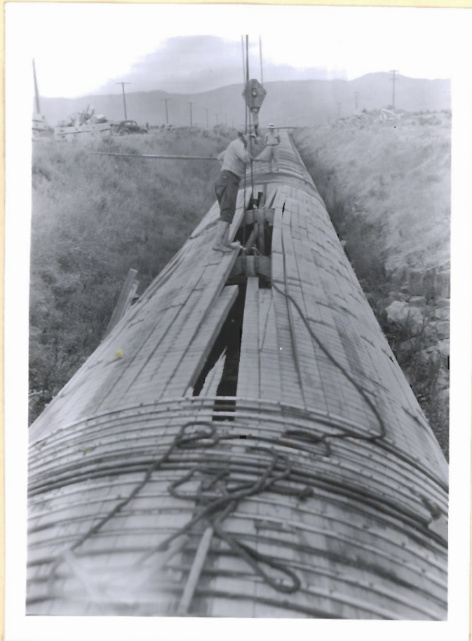
Foreman Leo Adams directing placing of templates in repair of collapsed pipe.
