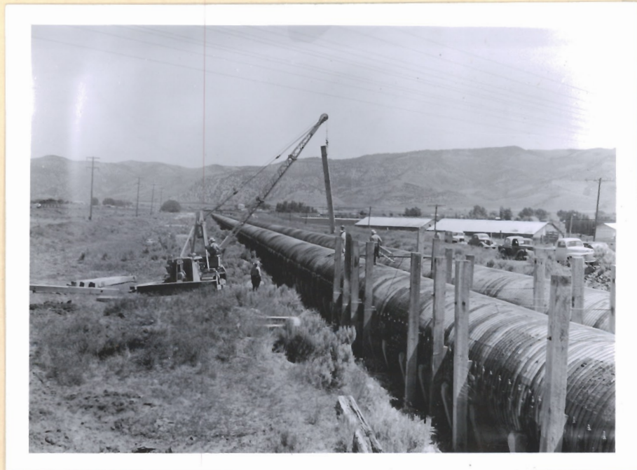
7-20-50 39019 #F-1 Erecting timber reinforcement on upper section of No. 2 Flowline. Timbers removed from section to be rebuilt in 1950. ER 48-1230.
