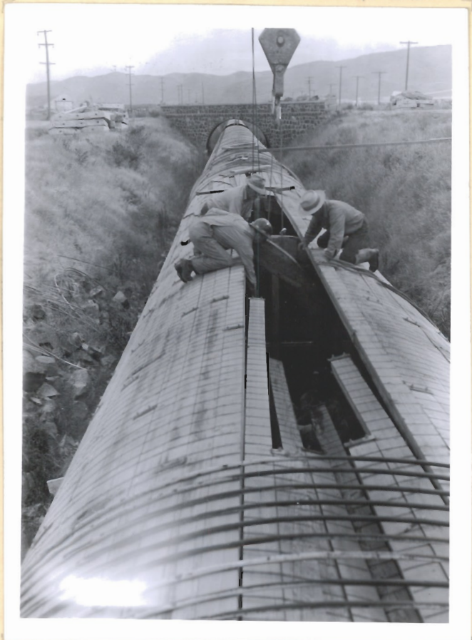
Shows workmen repairing section of pipe below highway bridge (1947 pipe construction) which collapsed due to vacuum created when pipe was drained to remove lower bulkhead of steel Wye (150 construction).
