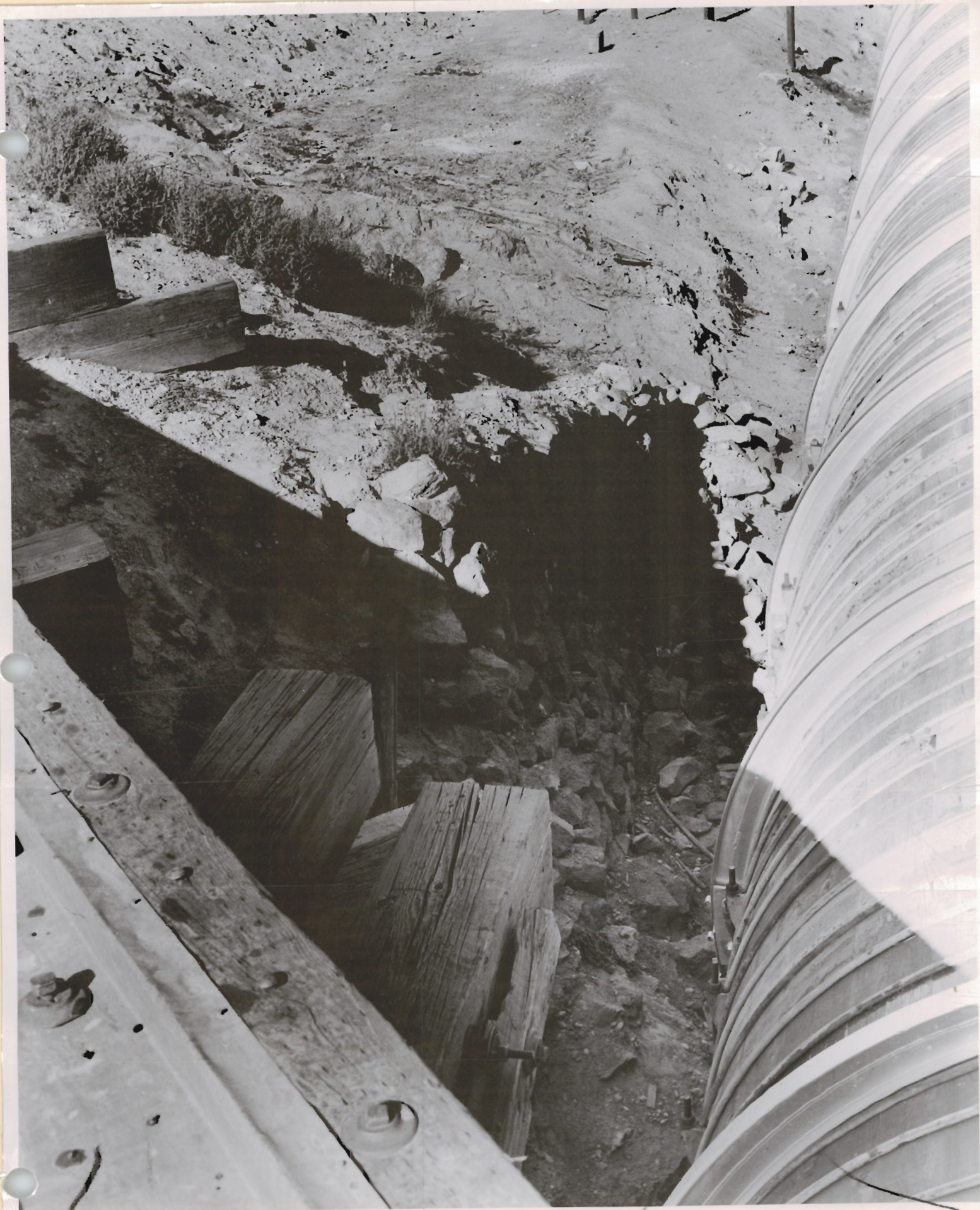
Title #2 UPRRCO. Bridge over Grace Flowline showing dry masonry wall east side of RR - No. side of pipe looking upstream - View from RR bridge.
