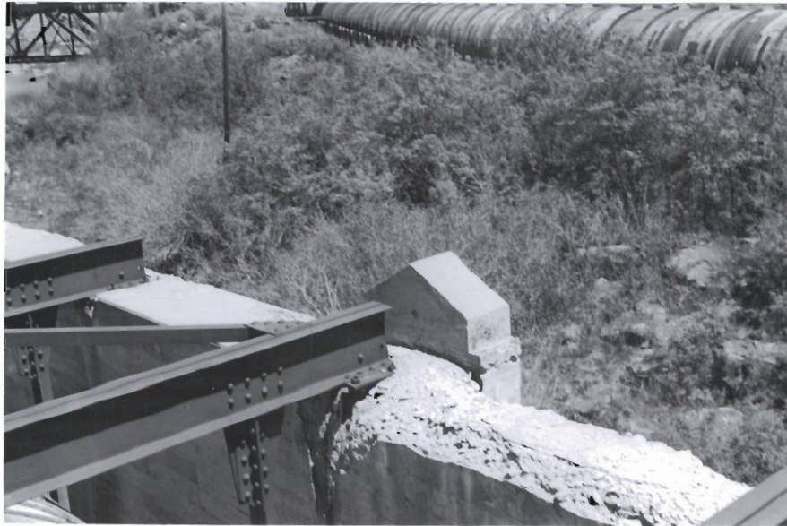
5. Showing deteriorated condition of concrete superstructure. 5-22-51
