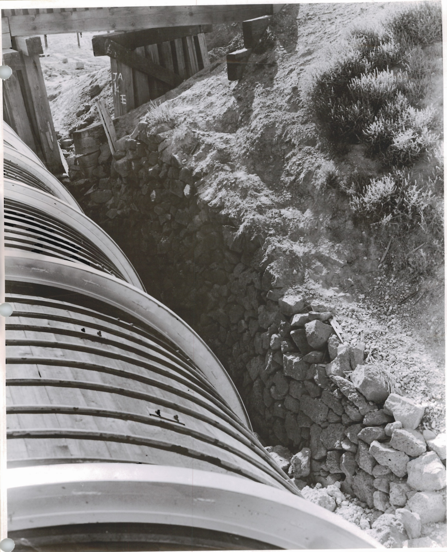
#3 UPRRCO. Bridge over Grace Flowline showing dry masonry wall east side of RR. No. side of pipe looking down stream.
