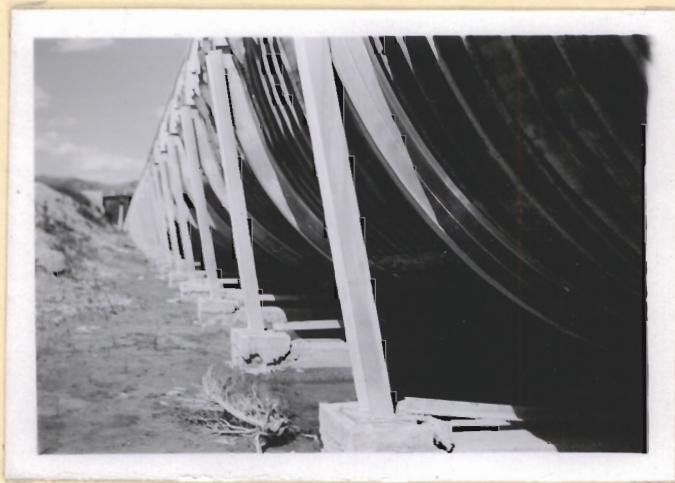
Looking Upstream. Showing bent lower member of saddle and fractured pad. 6--22-53
