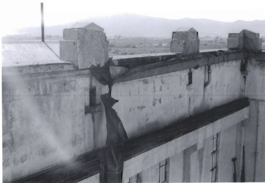
South wall inside after roof removal. Note deteriorated concrete. 9-26-57
