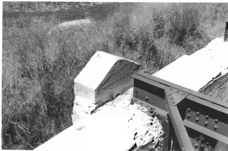
8. Showing deteriorated condition of concrete superstructure. 5-22-51
