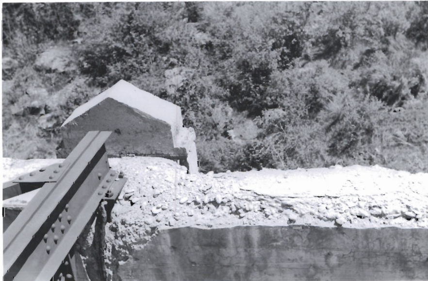
6. Showing deteriorated condition of concrete superstructure. 5-22-51
