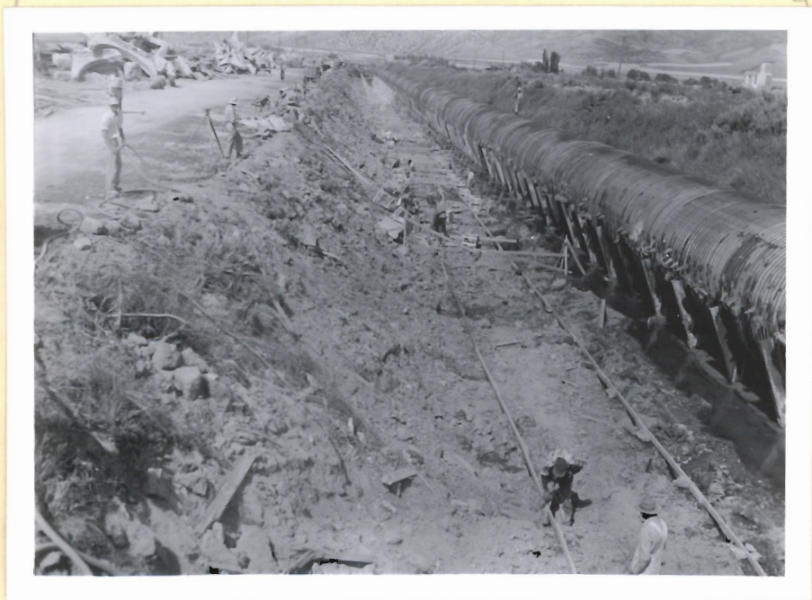
8-8-50 39026 Shows grade after removal of old saddles. Forming for new footings in progress.
