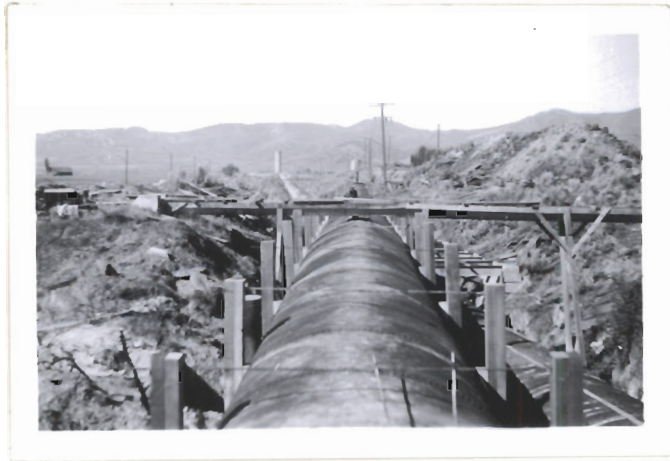
Collapsed section restored for filling. Note vertical braces with pillow blocks exerting pressure on sides thru tension rods top and bottom tightened with turn buckles to resist tendency to again flatten during filling. Filling started 7/27/48 1:50PM " completed " 7:05"
