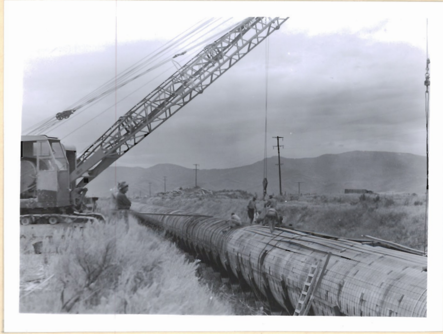
9-7-50 39032 #F-13 Crane used to place upper segment of template inside collapsed portion of pipeline.
