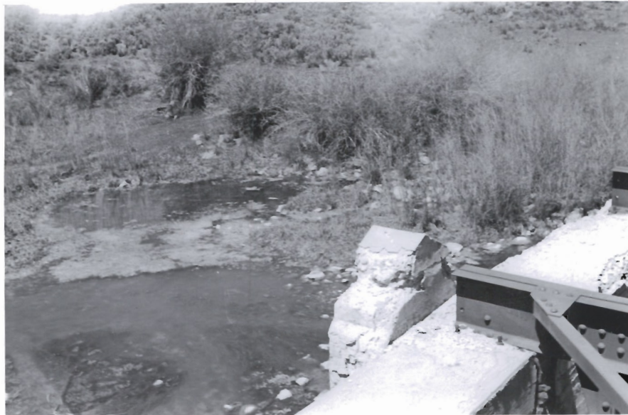
9. Showing deteriorated condition of concrete superstructure. 5-22-51 8th pilaster upstream on north side.
