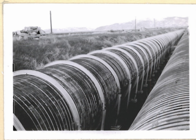
Showing bent saddle legs. 6-22-53
