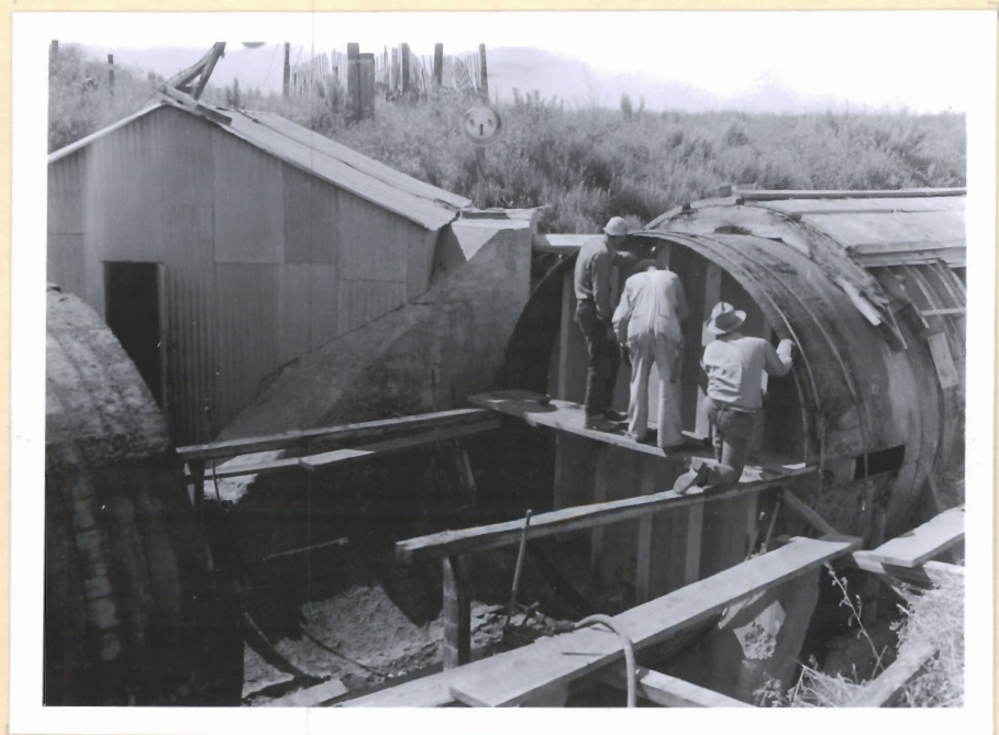
7-30-50 39020 #F-2 Installing steel bulkhead at Wye to permit use of lower section of flowline during reconstruction of the 6000 lin. ft. just upstream from the Wye.
