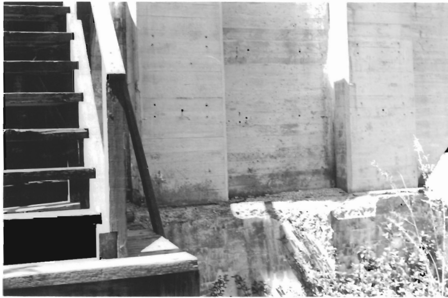
3. Showing deteriorated condition of concrete superstructure. 5-22-51
