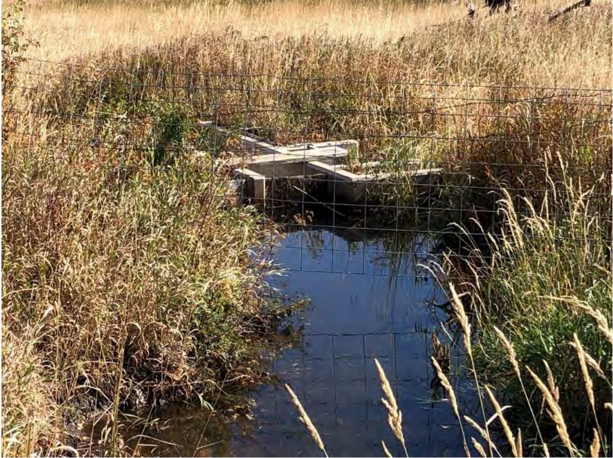
Alleman Lower Diversion Screening
