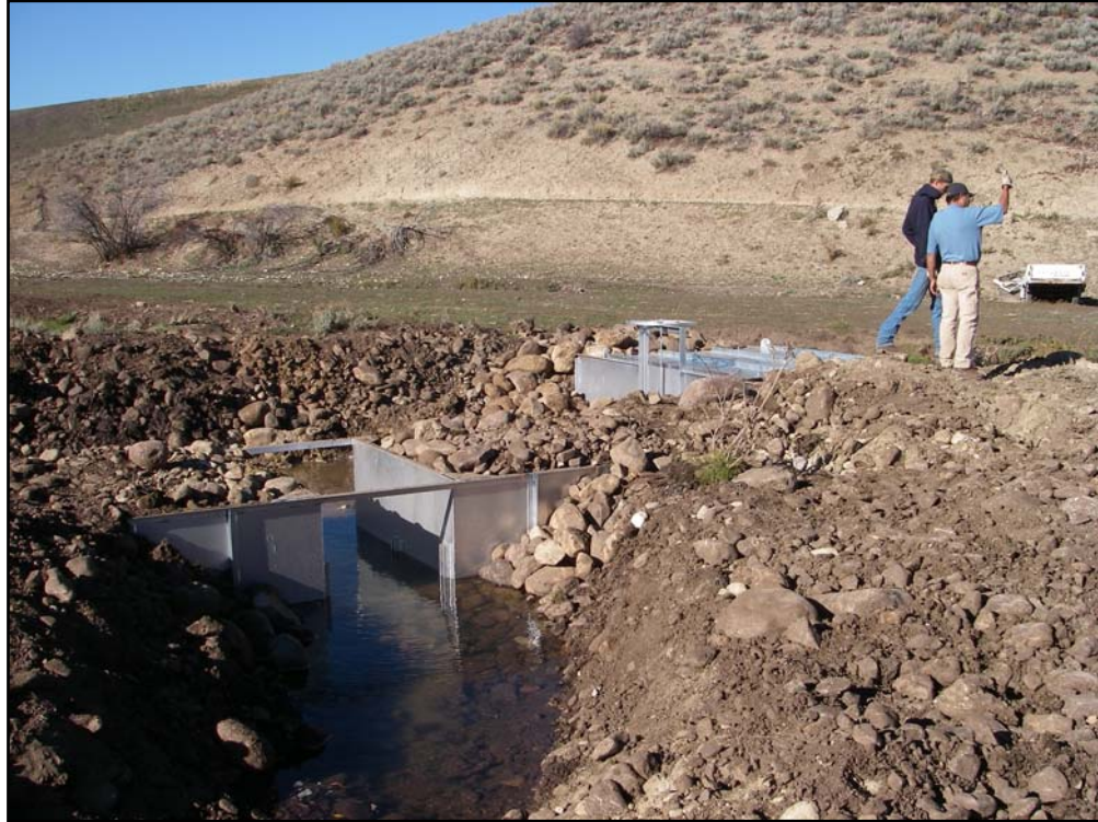
New fish passage and screening structures were installed at the Ovid irrigation diversion during 2006.
