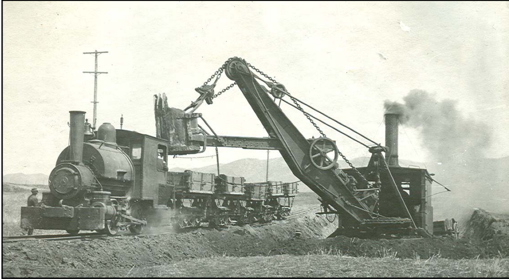
A small railroad track and engine used to transport materials at the Cove Hydroelectric Development construction site during the early 1900s.
