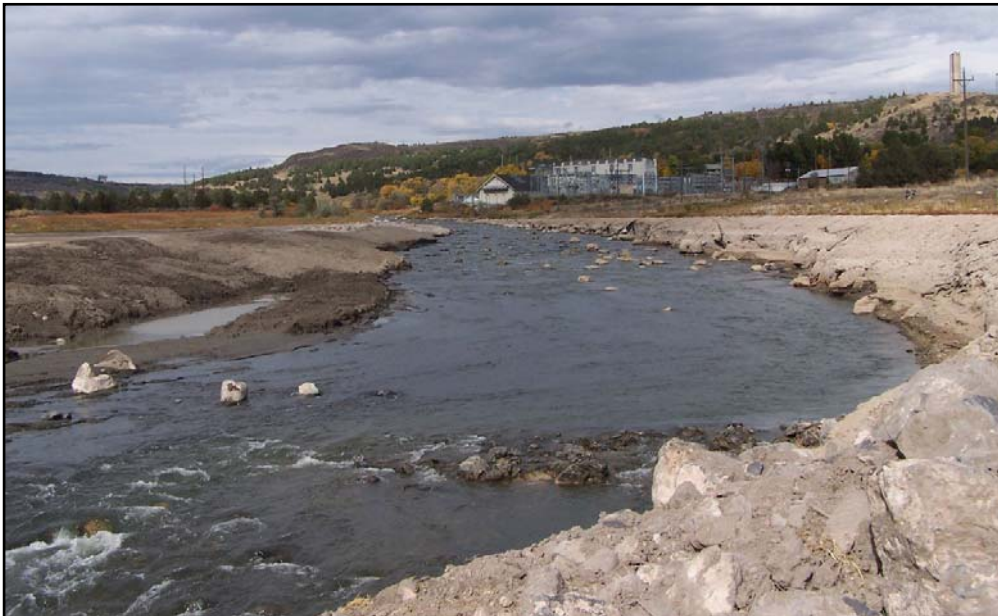
Bear River at the Cove decommissioning site following removal of dam in early fall 2006.
