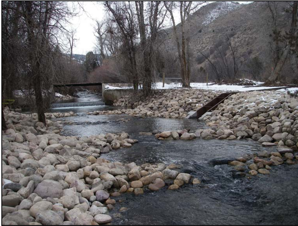
Cleveland Irrigation Company's diversion headgate on Cottonwood Creek was rebuilt during 2006 to prevent fish from being lost when water is diverted to irrigate fields. This habitat enhancement project was funded by the ECC in 2005.
