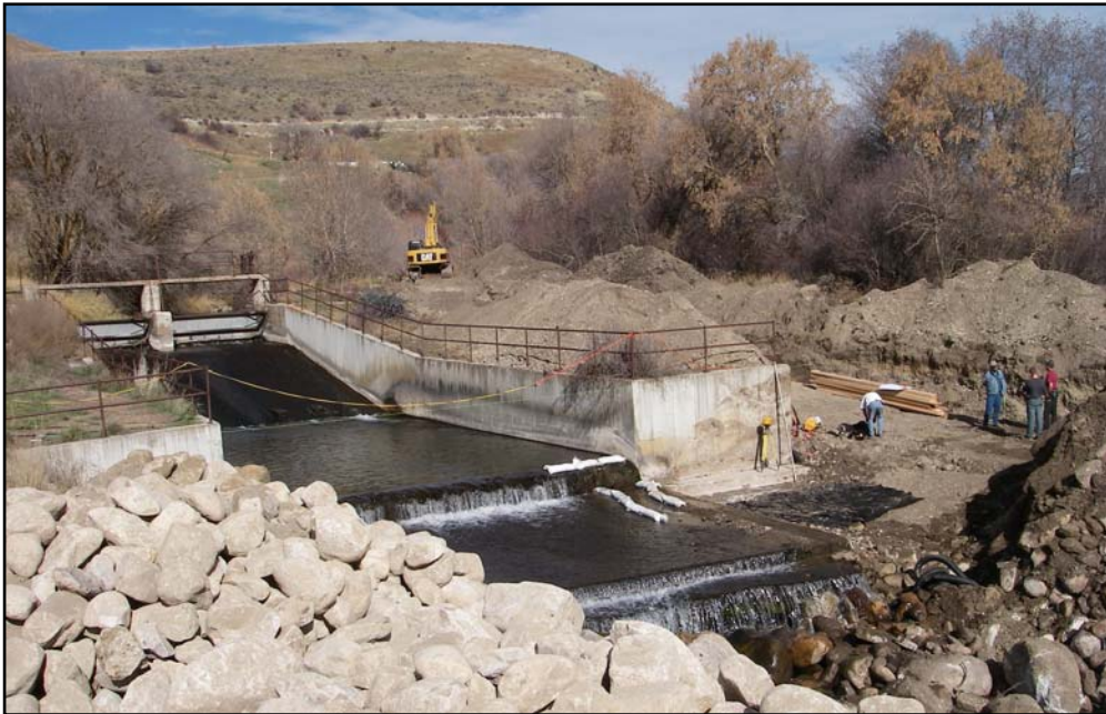
Fish passage and screening structures were constructed on the Cub River irrigation diversion near Preston, Idaho, during 2005 and 2006.
