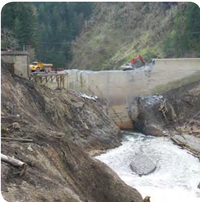
Demolition of the dam and facilities will continue through the summer months.
