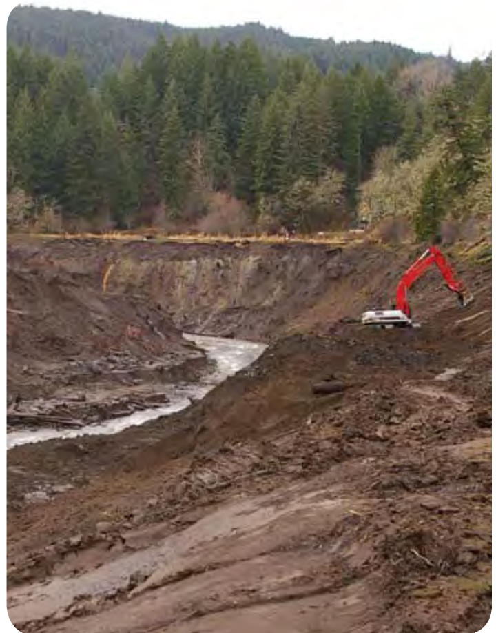
The grading of the riverbanks was done in the spring in preparation for fall hydro seeding.
