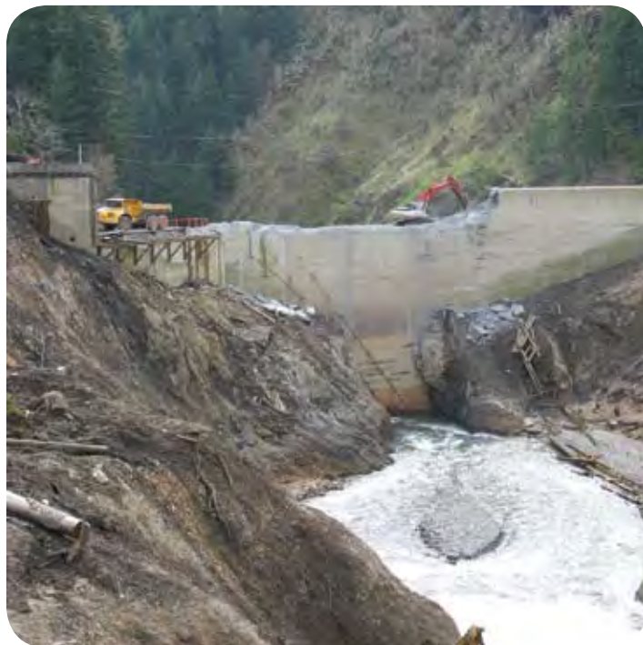
Demolition of the dam and facilities will continue through the summer months.
