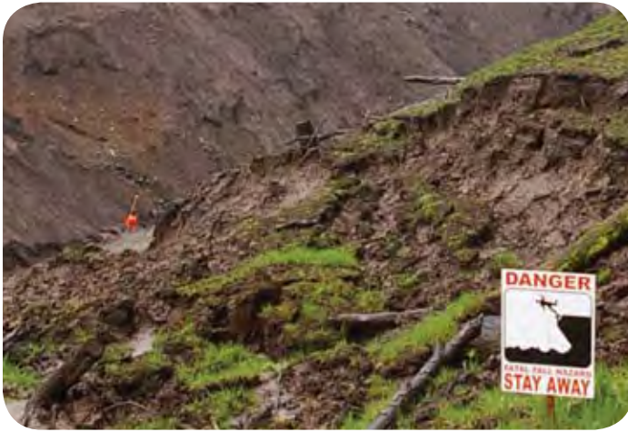
Public safety is PacifiCorp's top priority and we ask the public to obey all signs in the construction areas.
