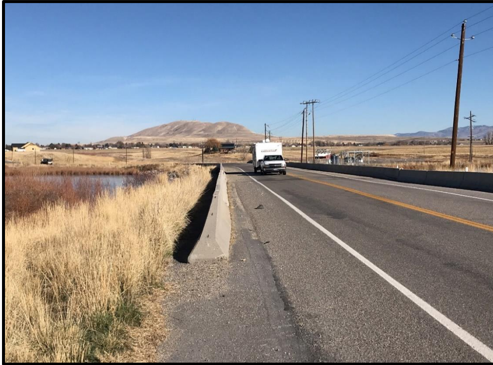
PHOTO 3-24 HIGHWAY 23 BRIDGE OVER CUTLER RESERVOIR NEAR NEWTON, UTAH, LOOKING NORTHEAST; LITTLE MOUNTAIN IS IN THE BACKGROUND
