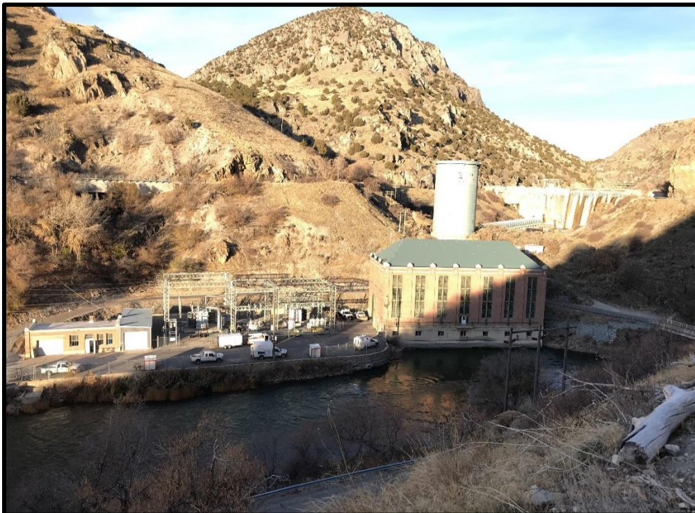
PHOTO 3-13 CUTLER POWERHOUSE AND SUBSTATION (NOT A PROJECT FEATURE), LOOKING UPSTREAM, CUTLER DAM AND CANYON IN THE BACKGROUND
