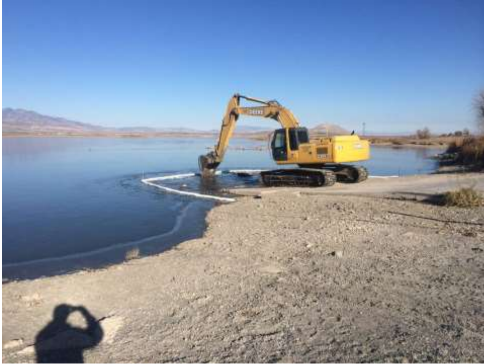
Photo D-7. Major ramp repair work at Benson Marina during reservoir draw down.
