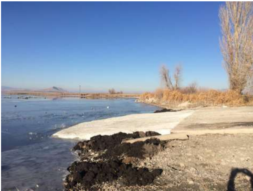
Photo D-6. Major ramp repair work at Benson Marina during reservoir draw down.
