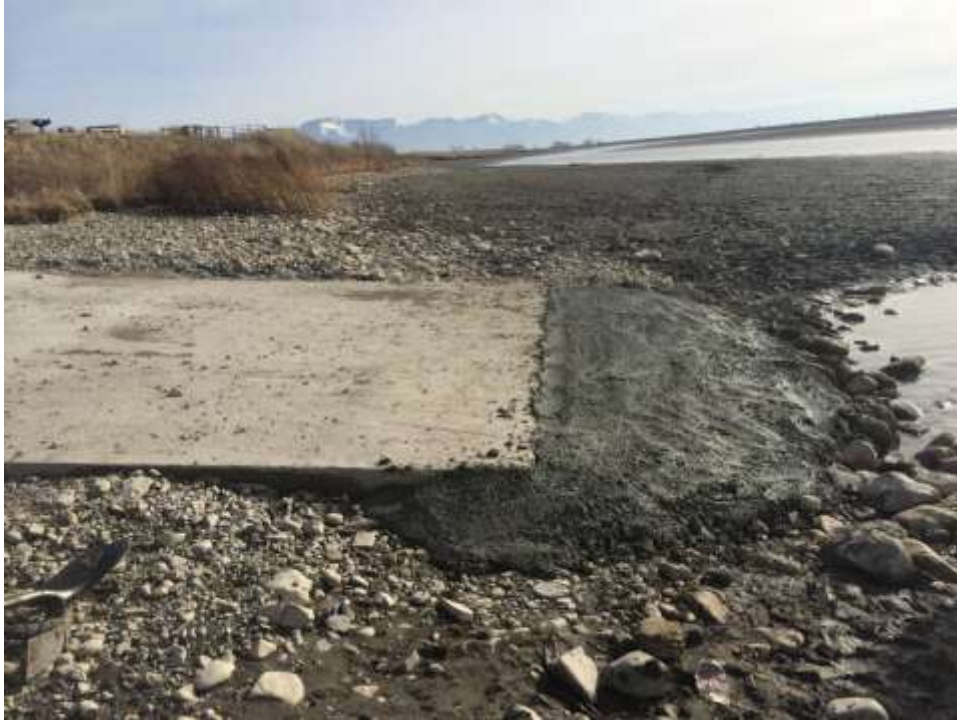
Photo D-5. Ramp repair work at Cutler Canyon during reservoir draw down.
