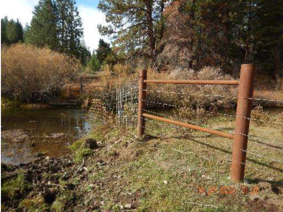
Figure 7. View of the southern intersection of Area 4 fence with Spencer Creek. H-braces were repaired and the cable was retensioned to establish proper hog fence positioning; new steel pipe bracing was installed on the far bank).
