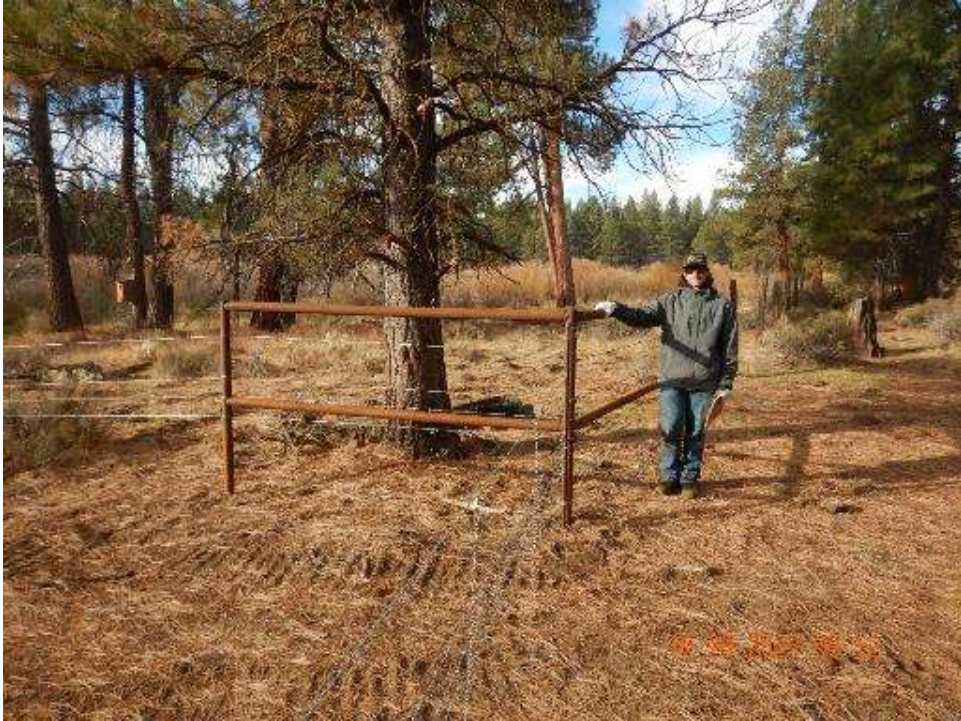
Figure 5. View of the northeastern corner of Area 2 fence. The aged wooden corner brace was replaced with steel pipe and the wires were retensioned and reset. New wildlife-friendly fence was installed leading to the northwestern crossing of Area 2 with Spencer Creek (visible at left side of the post-project photo).
