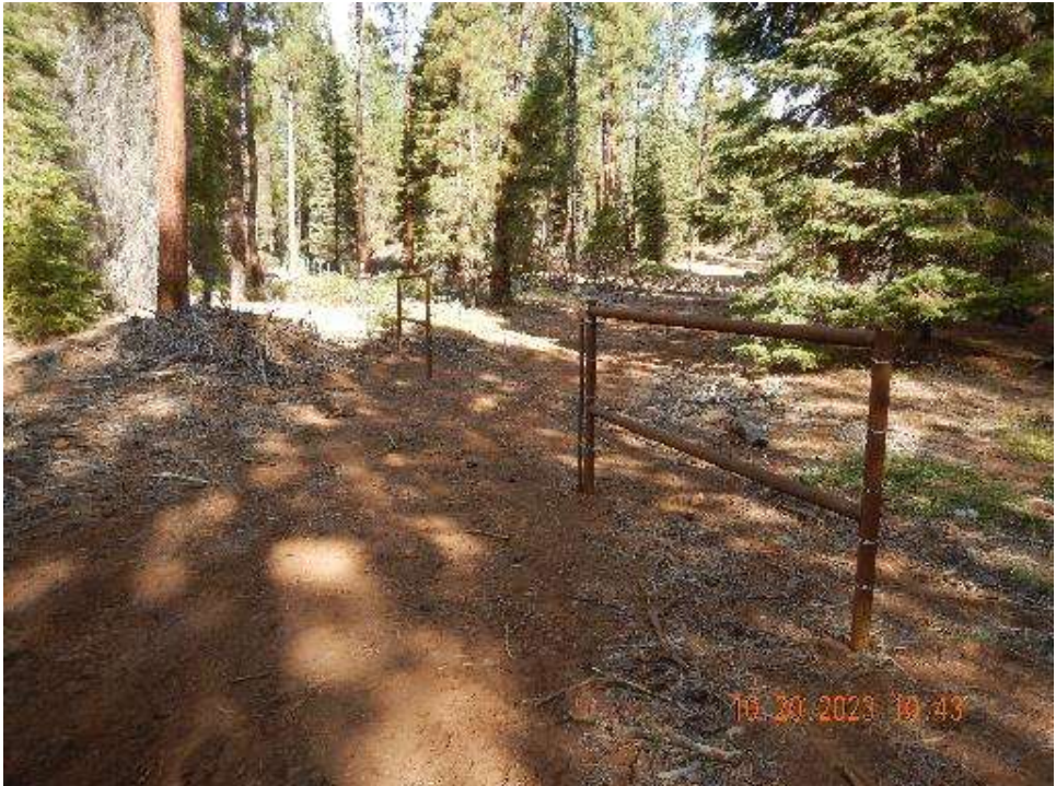
Figure 6. Location of new drive-through gate in southwestern portion of Area 4. Pre-project fence had been torn down to allow for passage on logging road; new drive-through gate with steel pipe bracing was installed allowing for vehicle access.
