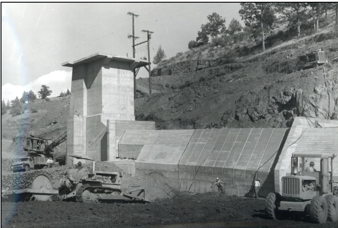
Figure 9. Outlet tower and waterway pipeline during construction (prior to control building construction). Picture is taken looking approximately to the southeast (source: PacifiCorp).
