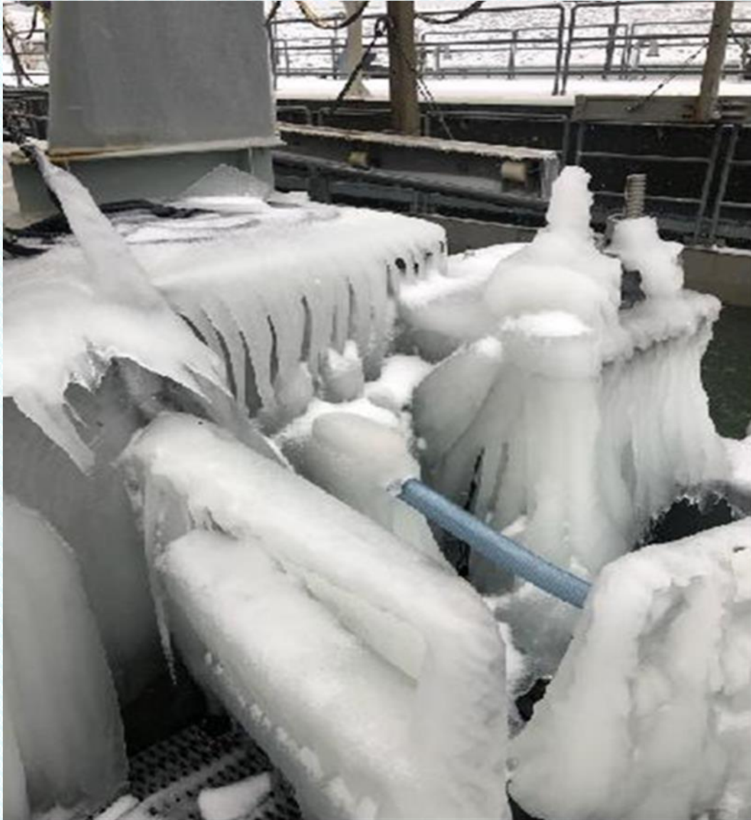
Figure 3. Ice accumulates on the Swift Floating Surface Collector during a winter storm in January 2024.
