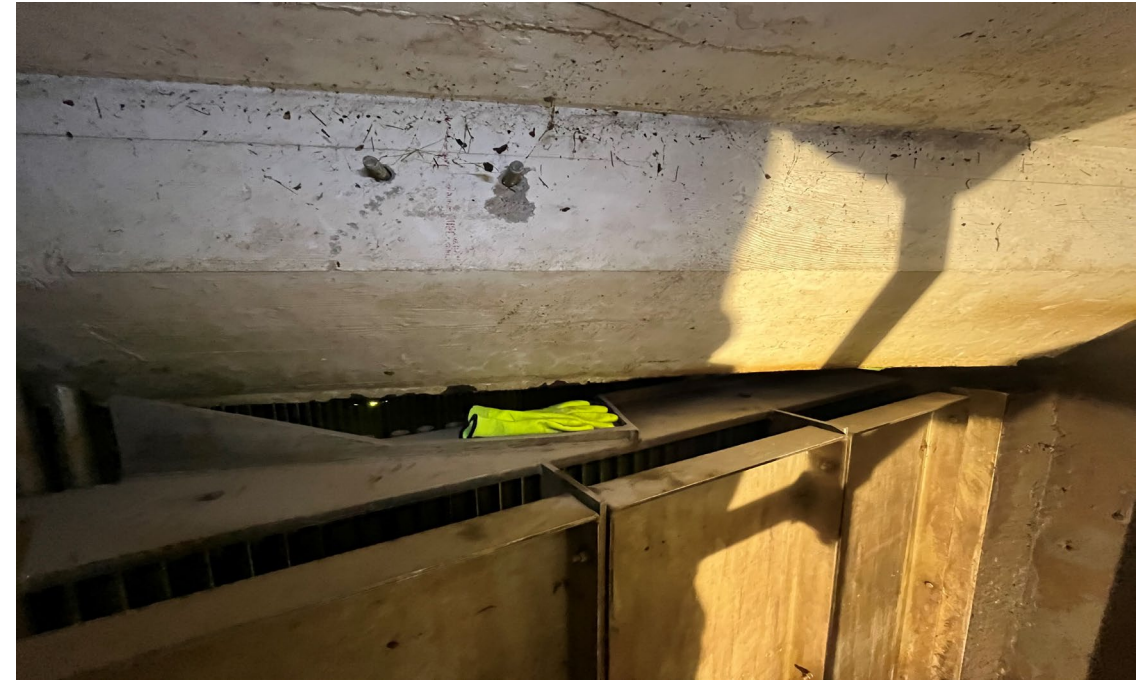
Original image of concrete void as viewed from the evacuation pump room – December 22, 2023.
