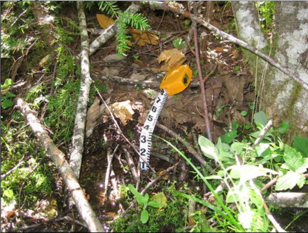
Blocked Culvert on FR9300150.
