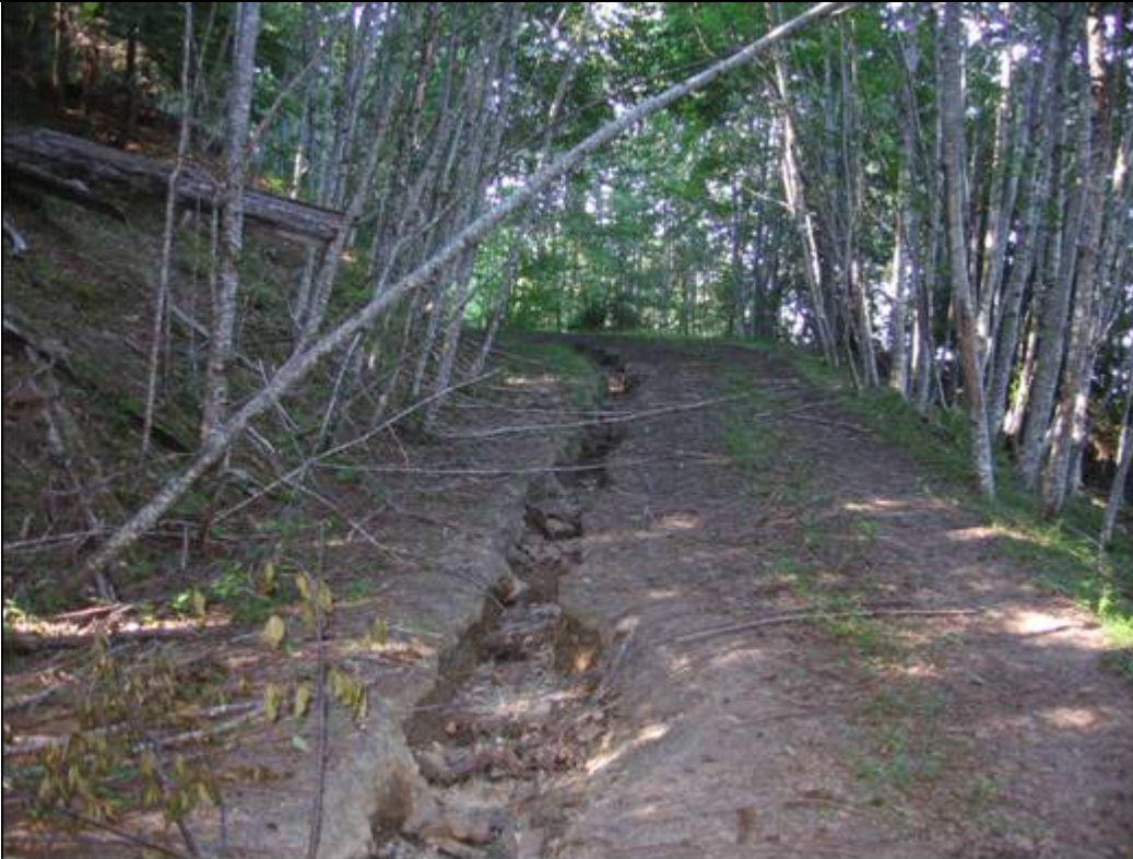
Surface erosion from blocked culvert on FR9300150.
