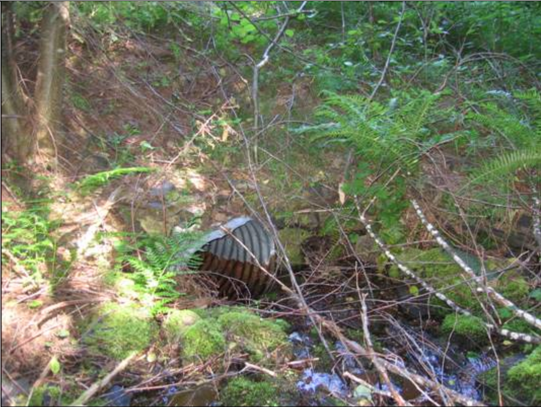
Collapsing culvert on FR930015.
