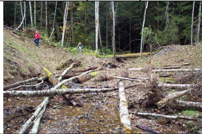
2008 Post – Project FR 8322700 Road Decommission – Road Fill Removed, Stream banks match adjacent natural slopes. Available large wood placed into stream and along stream bank, Trees still to be planted. Low gradient tributary to Muddy River.
