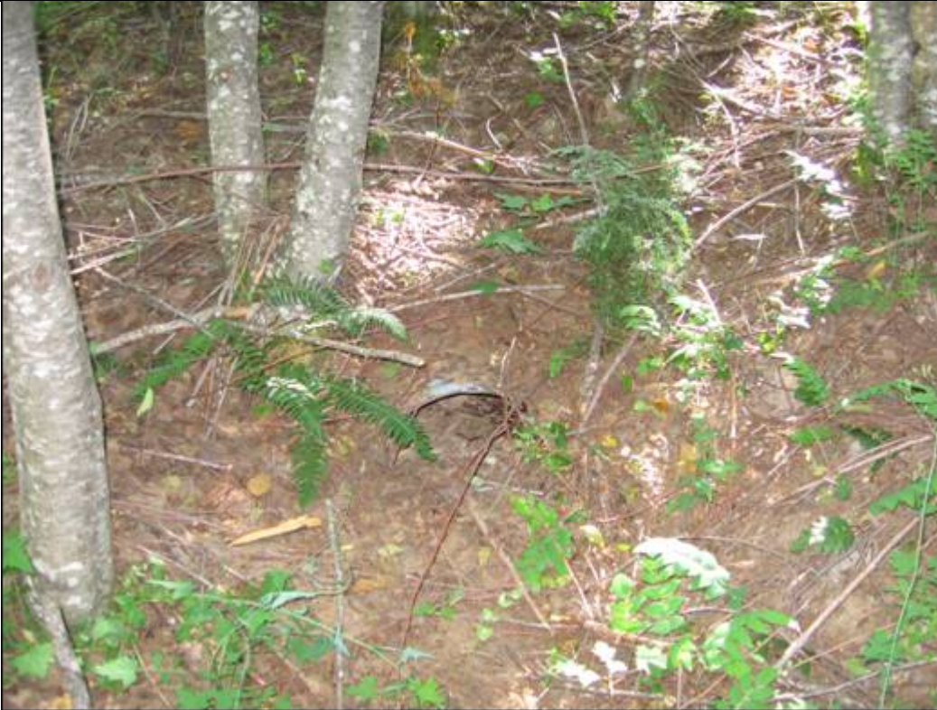
Blocked Culvert Inlet on FR9300150.
