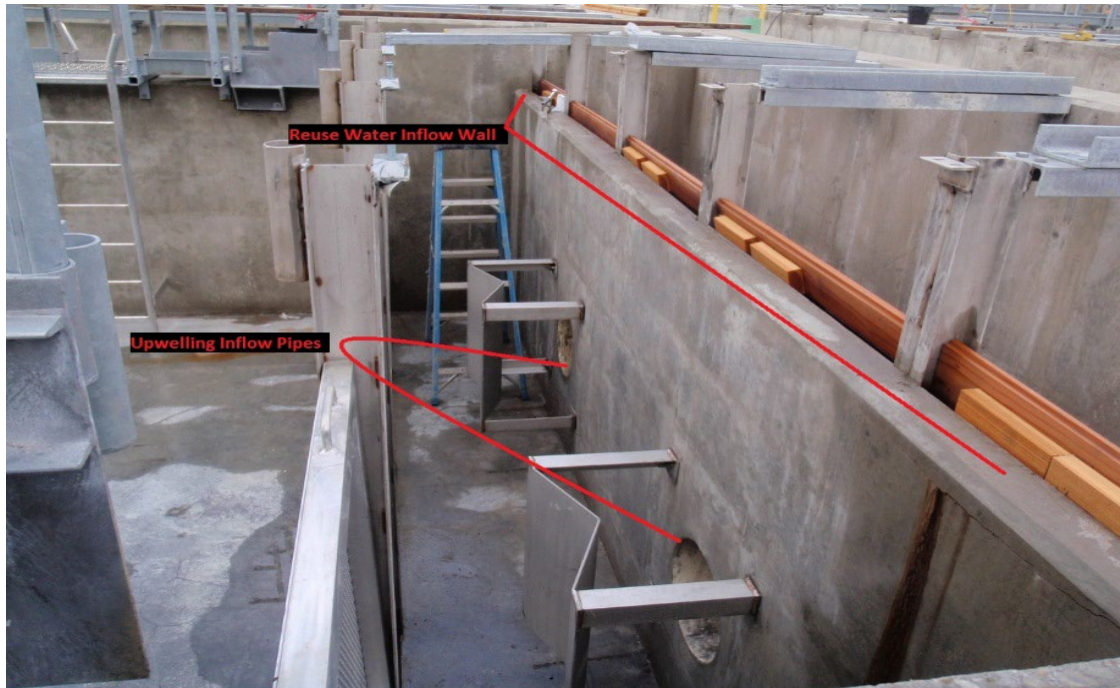
Figure 12. Photograph illustrating the overflow wall and first pass inflow pipes at raceway 14-1.
