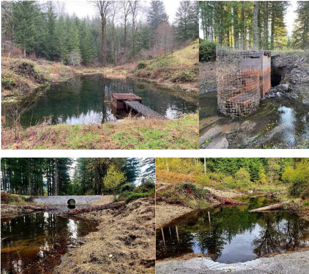
Figure 2. 8/12 Pond July 2019 before failure (upper left). Culvert failure February 2022 (upper right) final replacement of culvert 600C2 (lower left) the result for 8/12 Pond (lower right).
