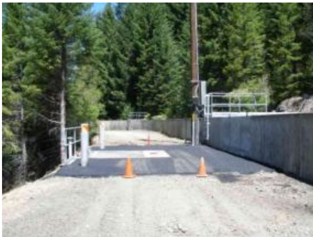
Fish Creek Canal Shut-off and Drainage System – Drain Site 2
