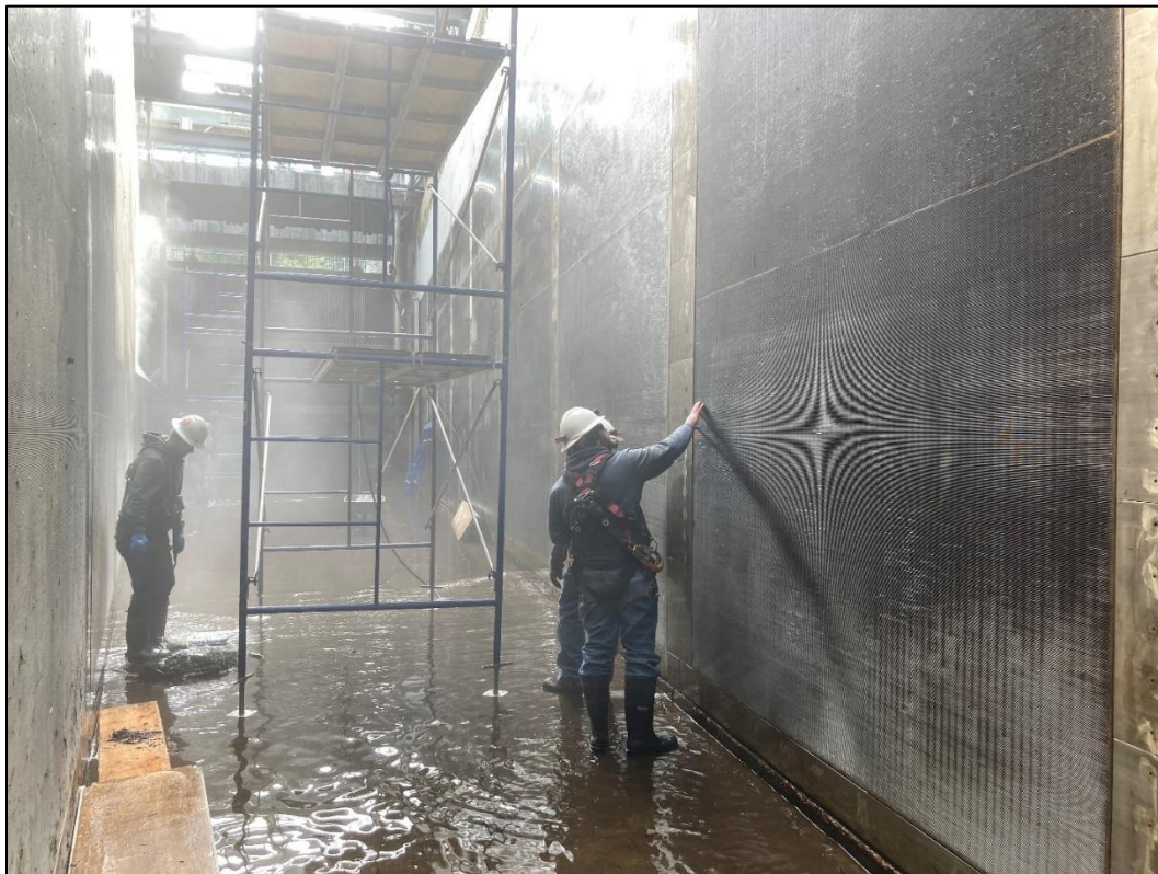
Figure 13. Cleaning and inspecting the Soda Springs Fish Screen while dewatered during a planned maintenance outage, February 2022.
