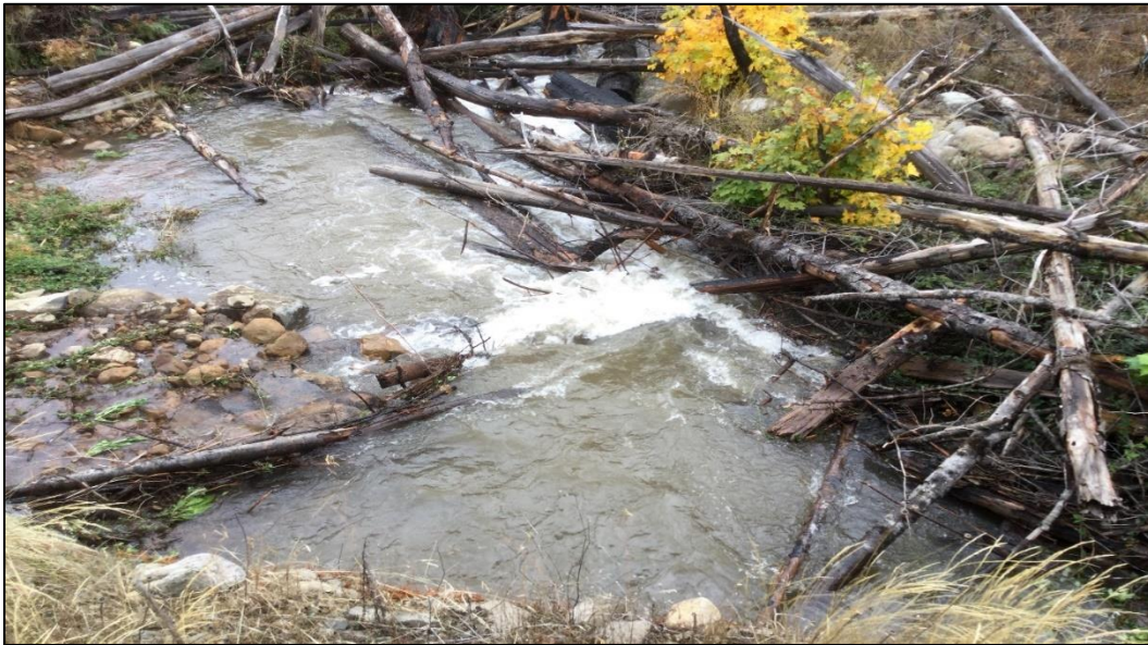
Figure 10. Boulders arranged to alleviate the 22” drop from Mace Creek culvert. Medium flow over the boulder tops provides small 5-6” steps for easy passage at all flows.
