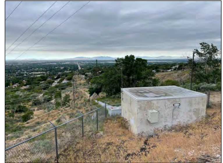
Pioneer PIV and Penstock
