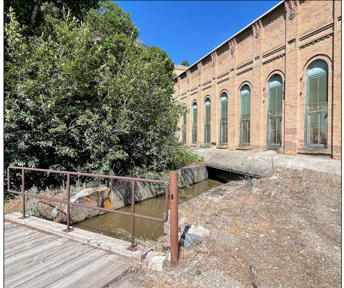
Granite Project's tailrace, which leads directly to the Big Cottonwood Water Treatment Plant
