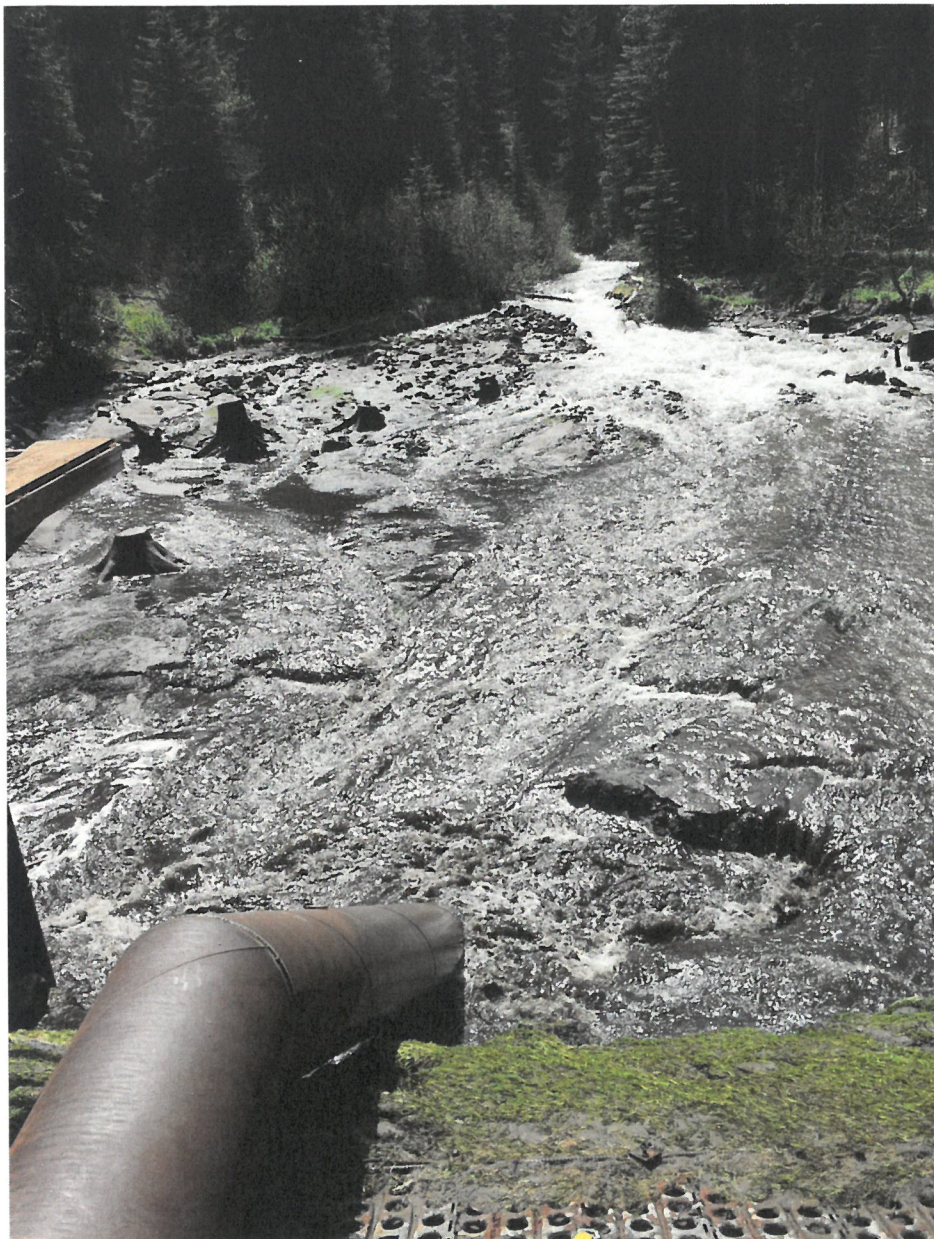
Photo 3 – 20-inch siphon in Wallowa Falls Forebay
