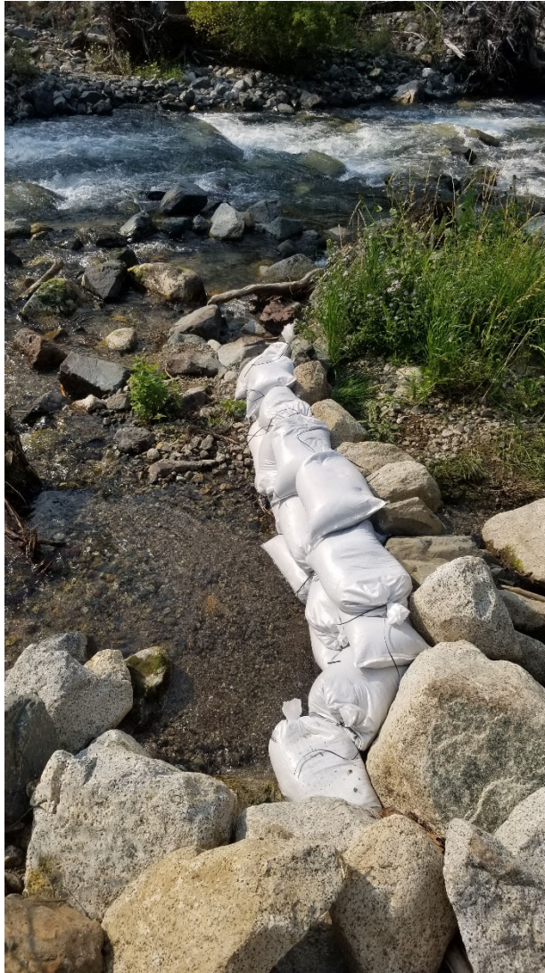
Figure 2. Photo of Wallowa Falls side-channel barrier on upstream end.
