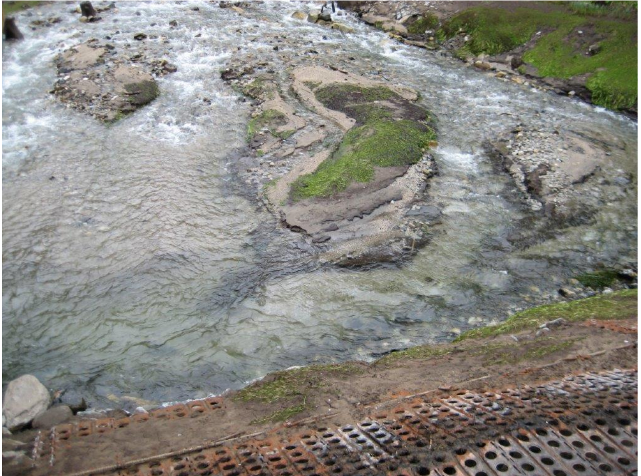
Photo 1 –Wallowa Falls Forebay – some sediment cutting along edges during draining on June 11, 2021
