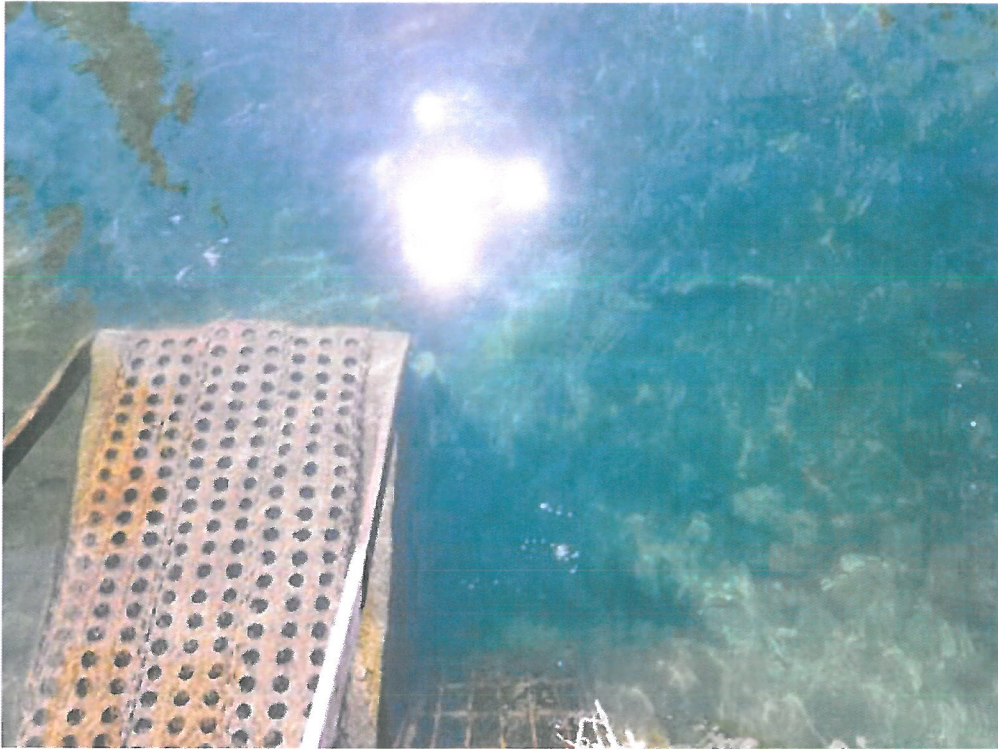
Photo 7 – Penstock intake and low level outlet trash rack after dredging and flushing operation
