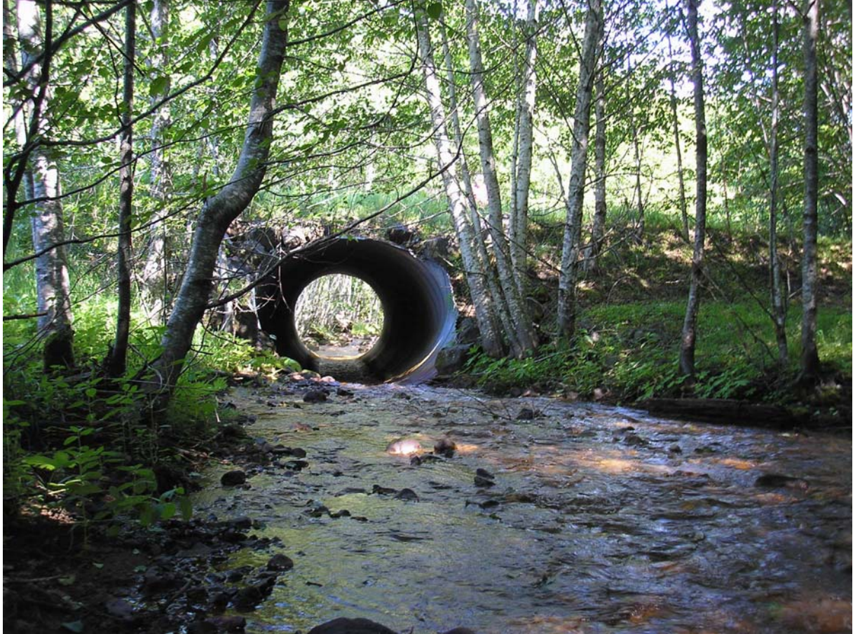
Picture 3. Culvert before replacement. Note kinked tree on left. Tracy 2005
