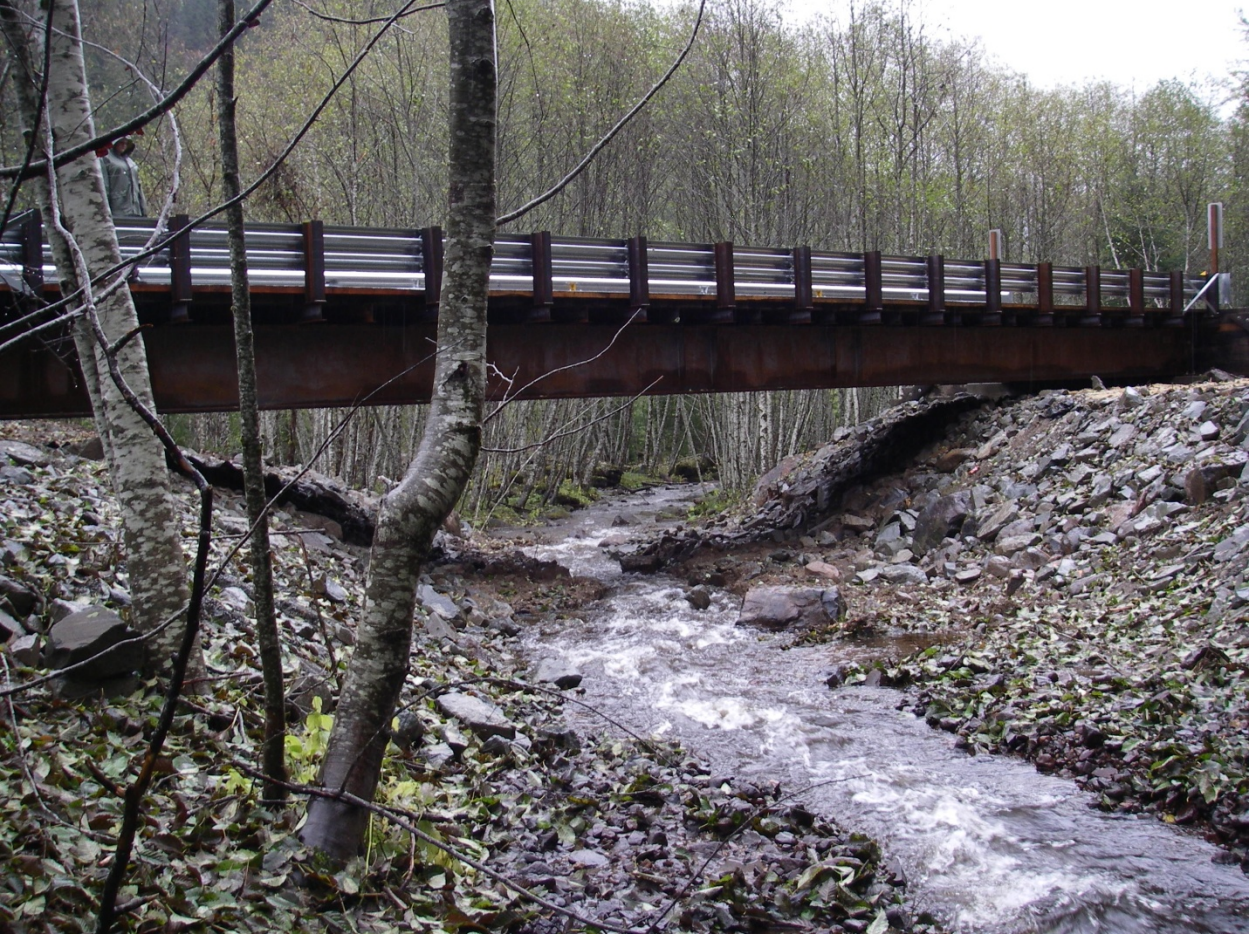
Picture 4. New bridge has replaced the culvert. Note Kinked tree on left. Becker 10/2009
