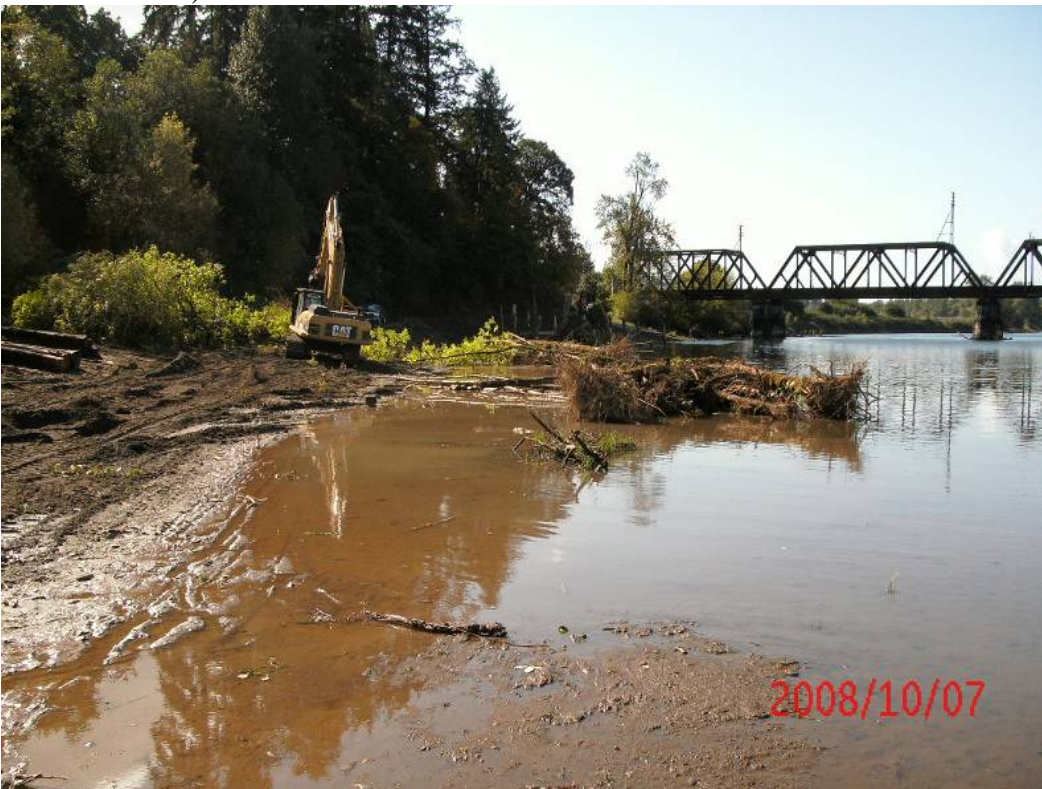
Wood debris being staged during low water times on site (Photo: Tony Meyer)
