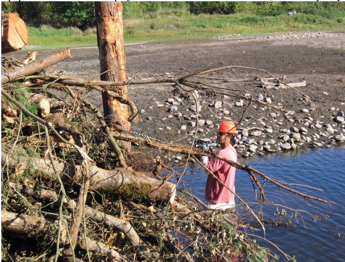
Holes were drilled into the pilings and structures to bolt and anchor each ELJ in place in order to prevent ELJ from floating out during high-water events. (Photo: Tony Meyer)
