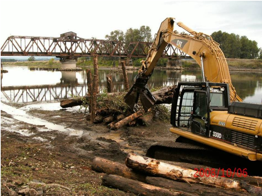
Pilings in place, and debris within the pilings, the boles are ready to be put into place. Land based equipment was used on this project because of the ease of access. (Photo: Tony Meyer)
