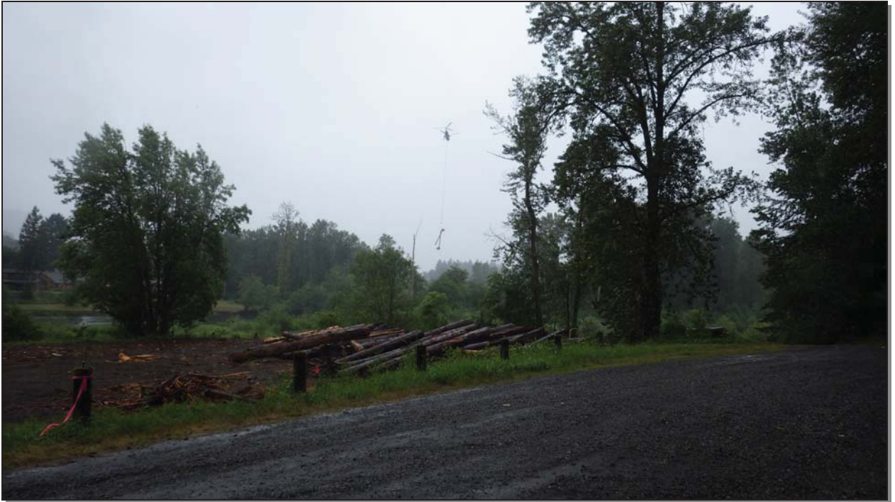
Columbia Helicopters lifted logs to Sites A and B in late June 2014.
