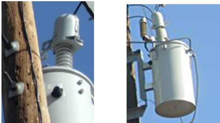
Figure 1—Station Service Transformer and Arrester Bird and Animal Protection
