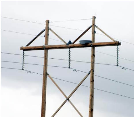
Problem nest relocated from above insulator string to nest tub
