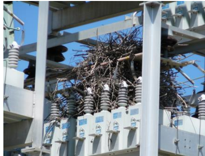
Problem nest in substation
